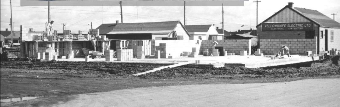
Constructing the Hornby Building which CBC moved into in 1962.... Now a Subway restaurant
